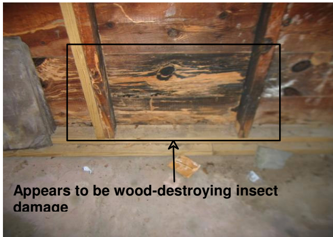
Figure Set - 13 There is evidence of wood-destroying insect damage on the rear & left side wall sheathing
