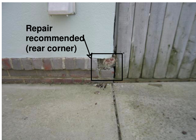
Figure Set - 7 A few areas of the brick foundation wall have missing bricks and mortar requiring repair
